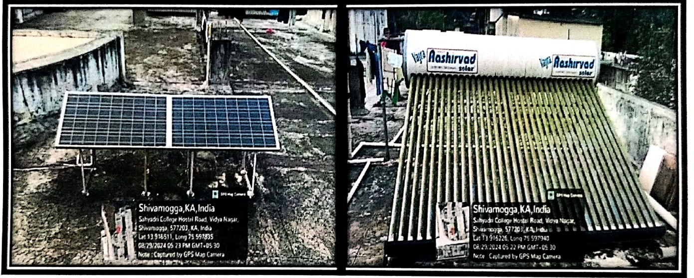
Solar Panels and Solar Water Heater installed at Hostel
